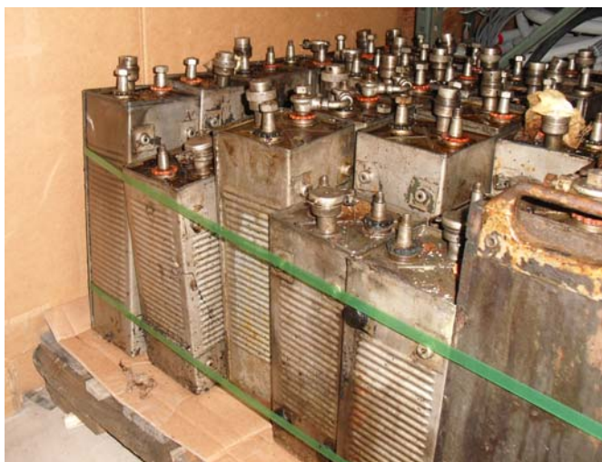
Picture 1. This shows the general condition of some of the cells as we received them.
